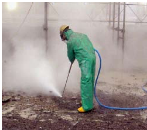
Stringent testing on-going in a Hydro demolition environment. No problems after 7 months of use
